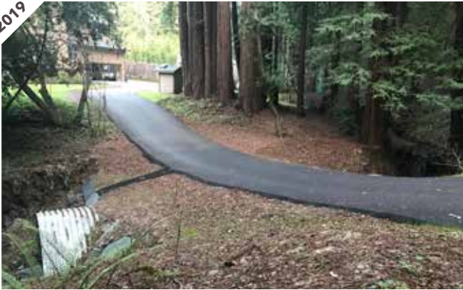
Photo point 1B: Banks are stable and the culvert is functioning as intended.
