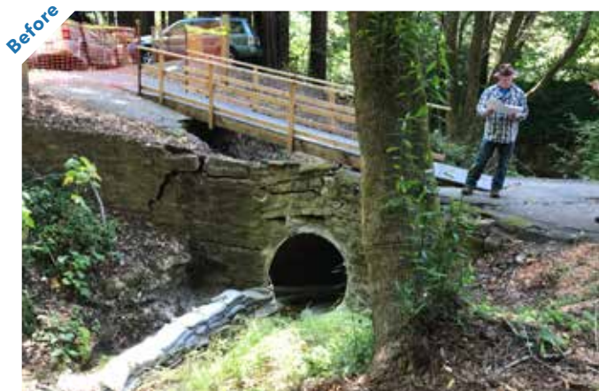
Photo point 3B: Looking downstream at the failed crossing.
