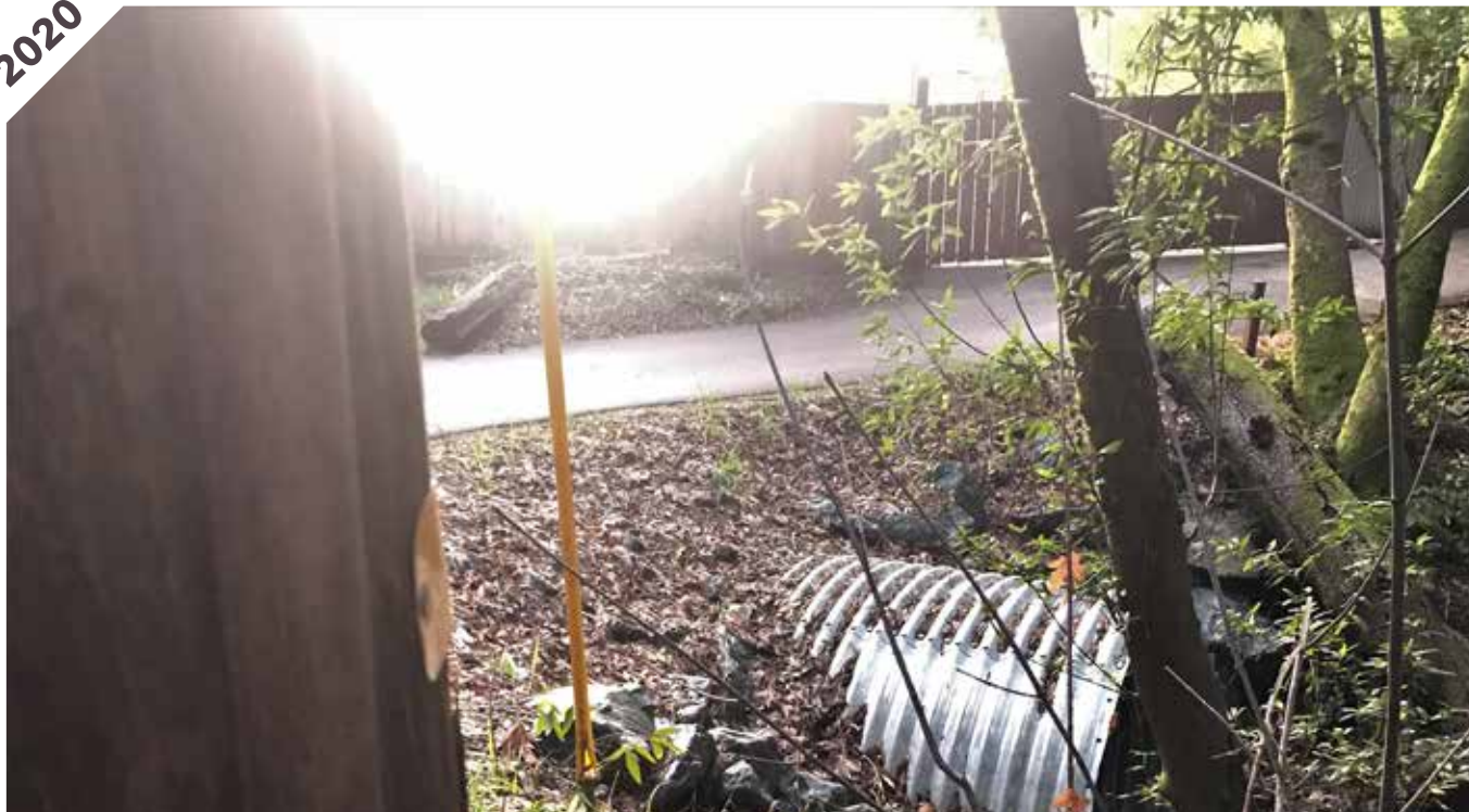
Photo point 3A: Looking downstream. The culvert is functioning well and no erosion is present.
