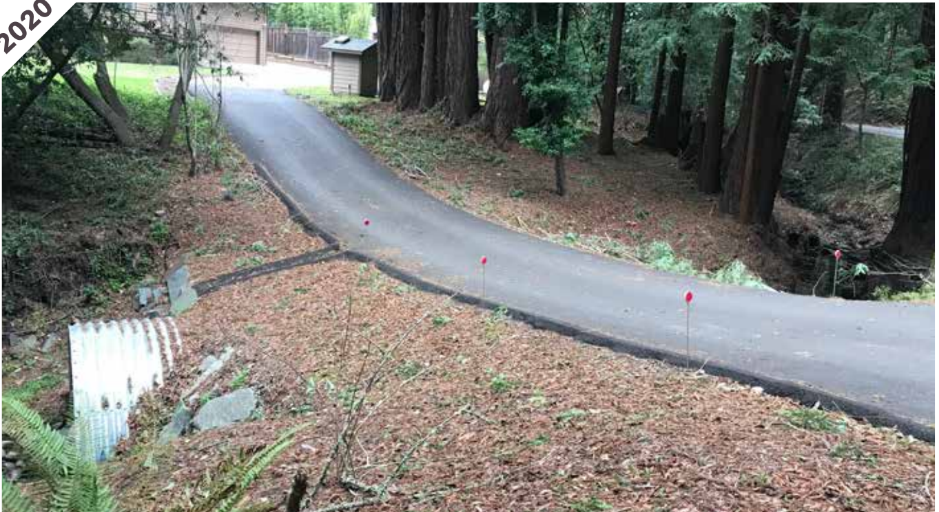
Photo point 1B: Looking upstream. Banks are stable and the culvert is functioning as intended.
