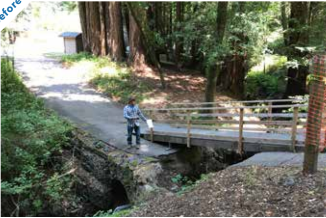
Photo point 1B: Looking upstream at the lower failed crossing.
