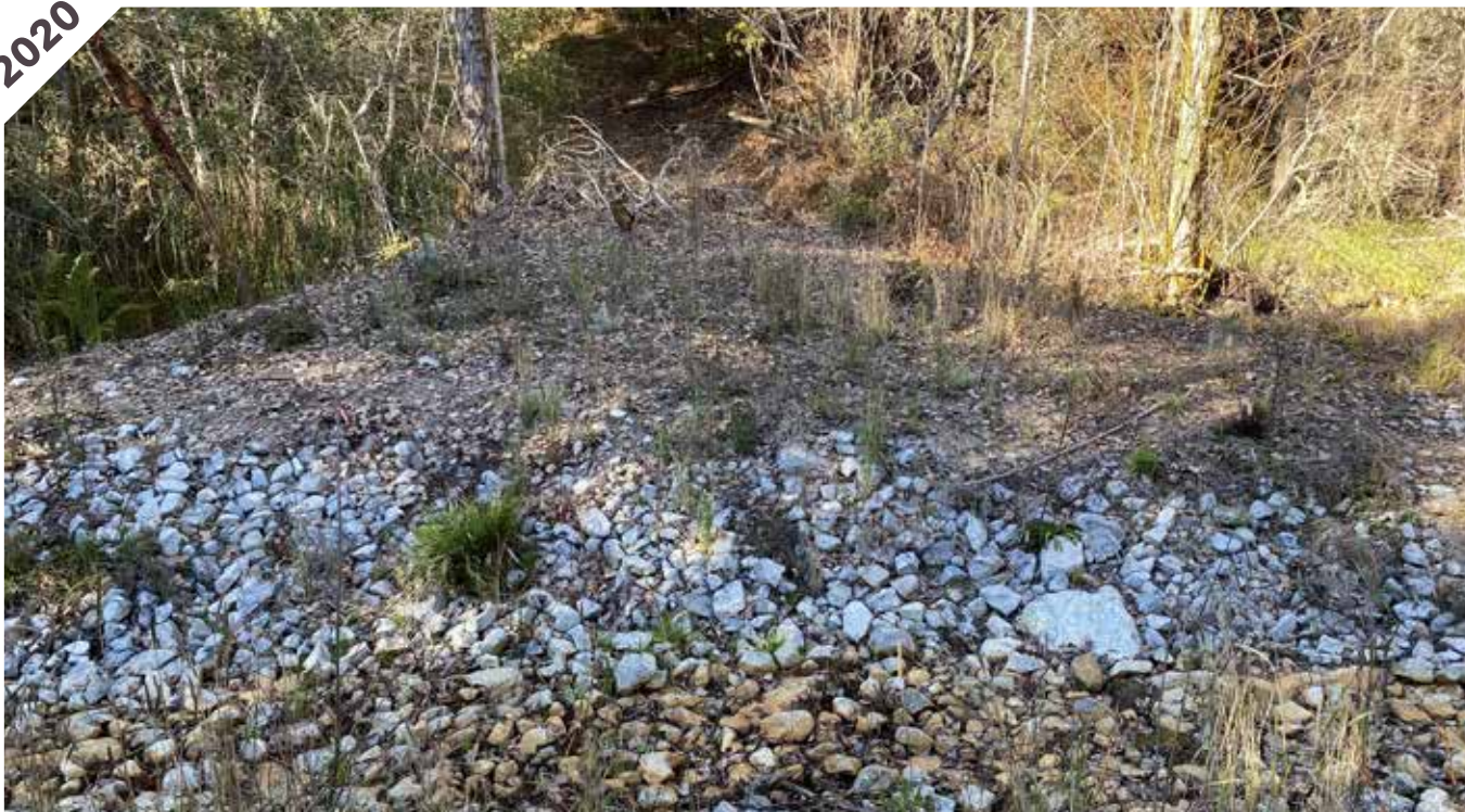
Photo point 3: Standing on the embankment and looking north, the rock lined channel is stable and the project area is becoming revegetated with willows and herbaceous vegetation.
