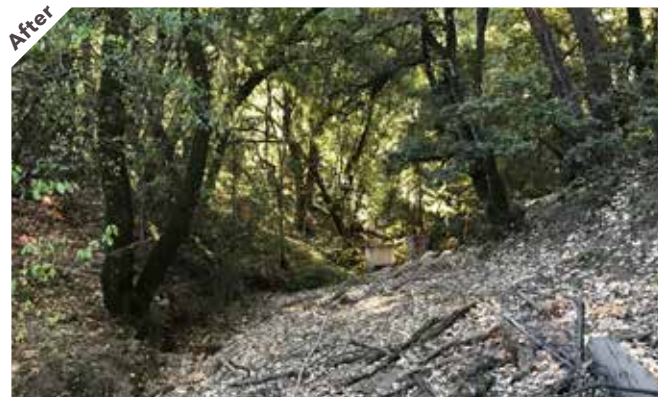
Photo point 2: The road was outslopped to closer mimic the natural slope of the land. Wood debris and understory duff removed during construction was spread back over the area.
