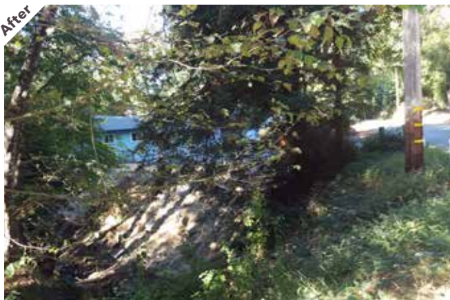
Photo point 5: Looking north. The plastic has been replaced and the bank repaired.
