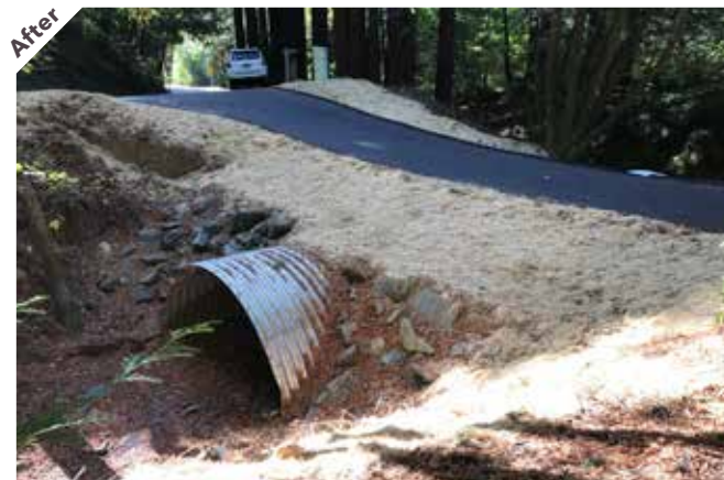
Photo point 3B: Looking downstream at the new crossing sized and placed for improved fish passage.
