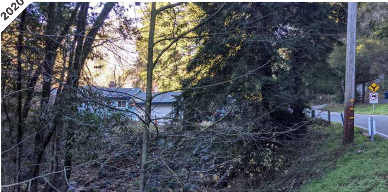
Photo point 5: The bank repaired has been repaired with the rock barely visible due to duff and native plantings.
