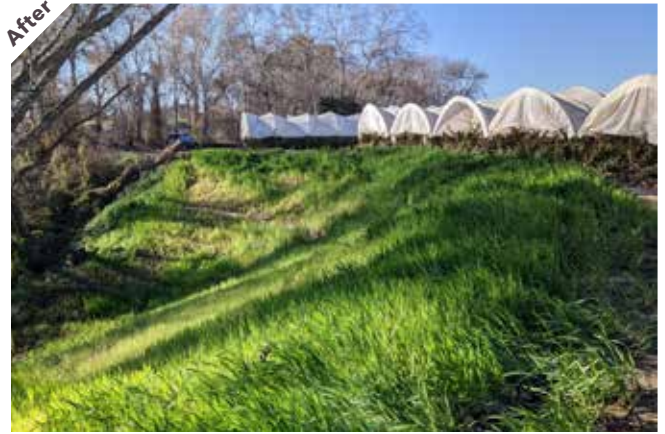
Photo point 1: Looking west, the bank has been excavated to a 2:1 slope. Fiber rolls have been installed along the contour and common barley is providing erosion control.
