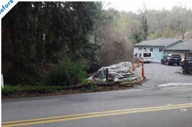
Photo point 3: Looking at the project site from across Branciforte Drive before project completion.
