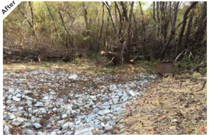
Photo point 1: Looking upstream, the culvert has been removed and replaced with a rock-lined open channel.
