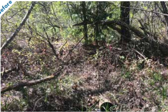
Photo point 4: Looking downstream, the inlet to the undersized culvert to be removed is visible.
