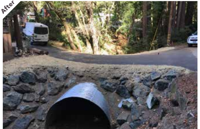
Photo point 1A: Looking upstream at the new, fish friendly crossing and repaved road.
