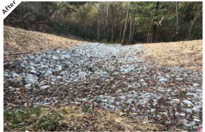
Photo point 4: Looking downstream, the culvert has been removed and replaced with a rock-lined open channel.
