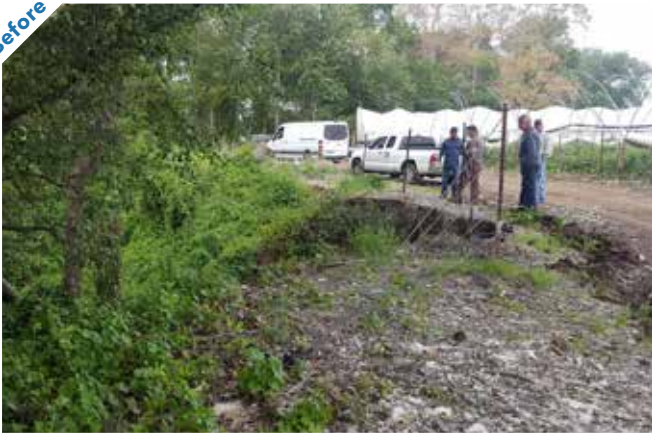
Photo point 1: Looking west at the eroded streambank, which has a nearly vertical slope.
