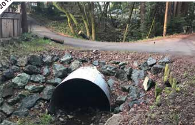
Photo point 1A: The engineered stream materials in the culvert has stayed in place and there is no erosion present around the culvert.
