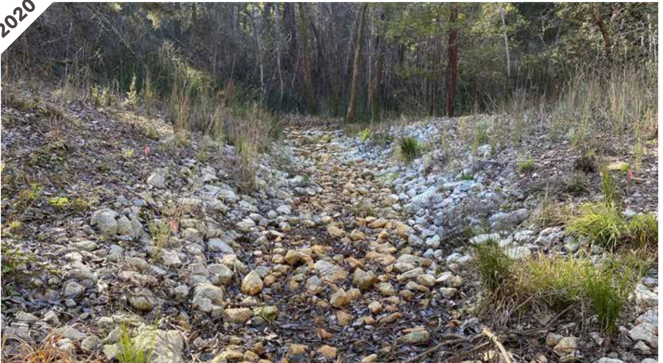
Photo point 4: Looking downstream, the rock-lined open channel that replaced the undersized culvert is becoming revegetated with willows and herbaceous vegetation.
