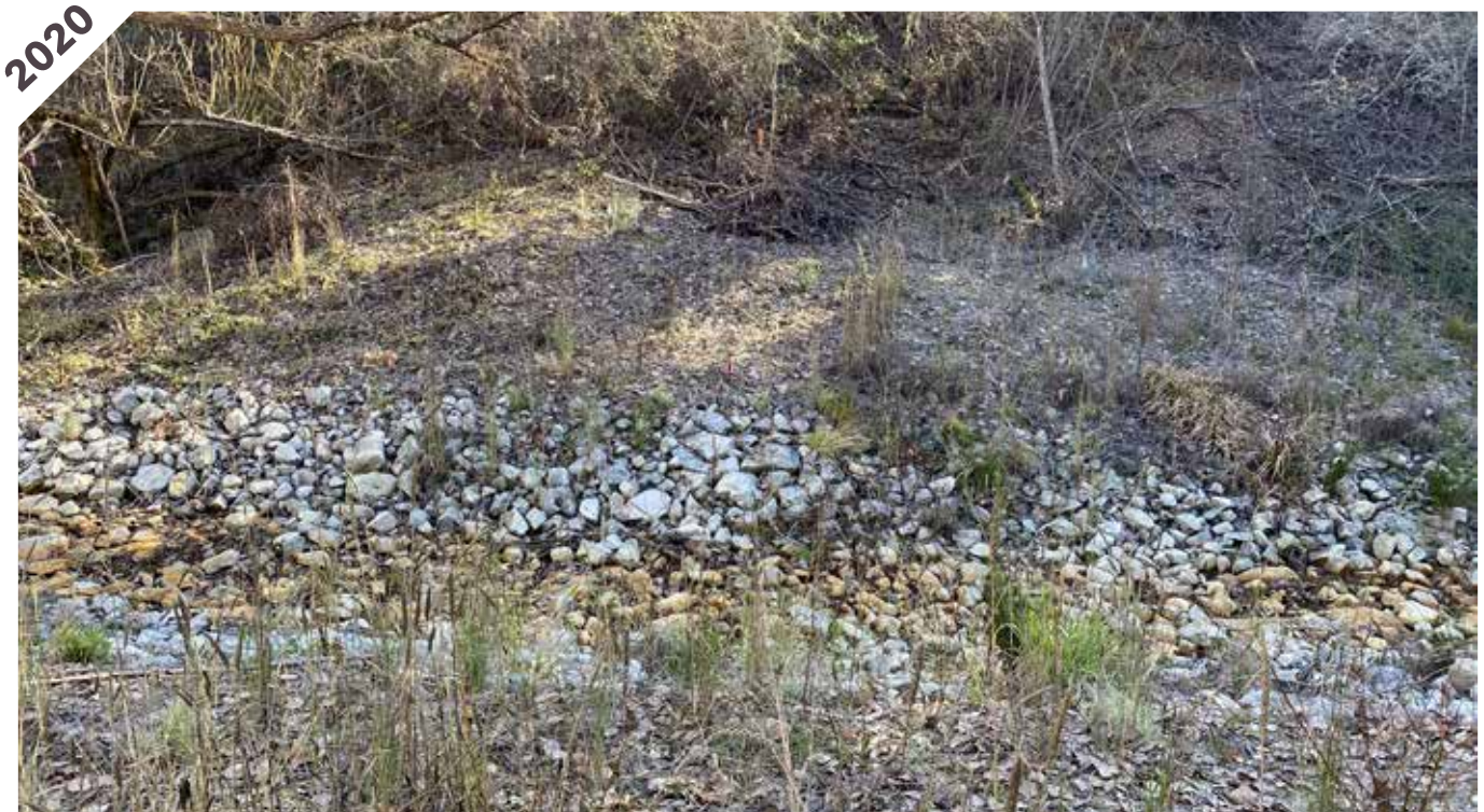
Photo point 5: Standing on the embankment and looking south. the rock lined channel is stable and the project area is becoming revegetated with willows and herbaceous vegetation.
