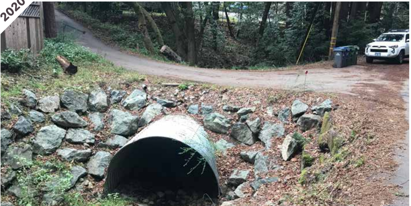
Photo point 1A: The engineered stream materials in the culvert have stayed in place and there is still no erosion present around the culvert.
