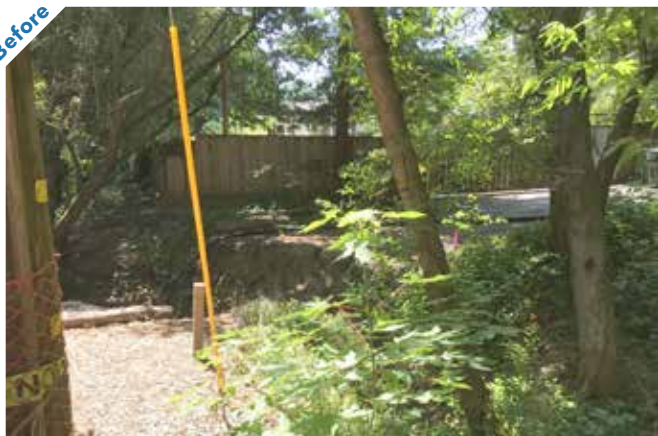
Photo point 3A: Looking downstream at the upper crossing failure.
