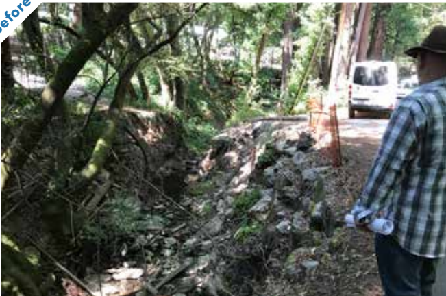
Photo point 1A: Looking upstream at the failed upper crossing from Mountain View Drive.
