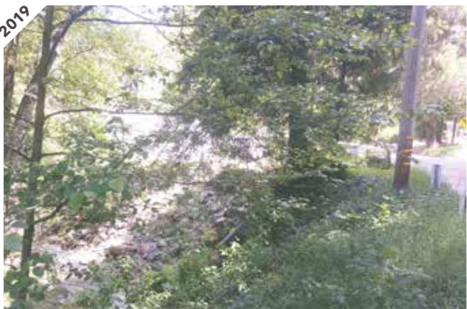
Photo point 5: The plastic has been replaced and the bank repaired observed on the far bank of Branciforte Creek.
