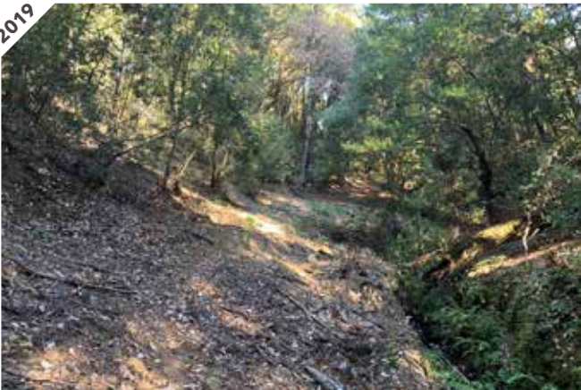
Photo point 5: Looking north at scarp failure. There is some slumping due to a natural seep. Landowner is monitoring.
