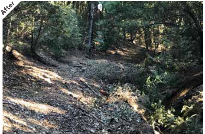
Photo point 5: The road recontoured to more closely match the natural slope on the left and prevent ponding or concentrated runoff. Understory duff was stockpiled during construction and spread back over the area post-construction.
