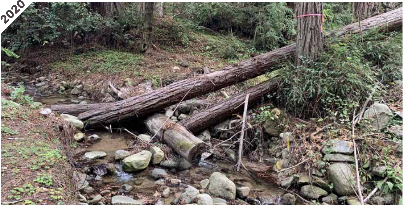
Photo point 5: The large wood and notch in the side channel has successfully diverted flow onto the floodplain, which has created a seasonal braided channel that runs roughly 300-400 feet downstream through the floodplain before rejoining San Vicente Creek.
