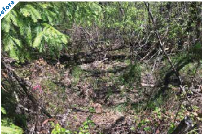
Photo point 1: Looking upstream, the inlet to the undersized culvert to be removed is visible.
