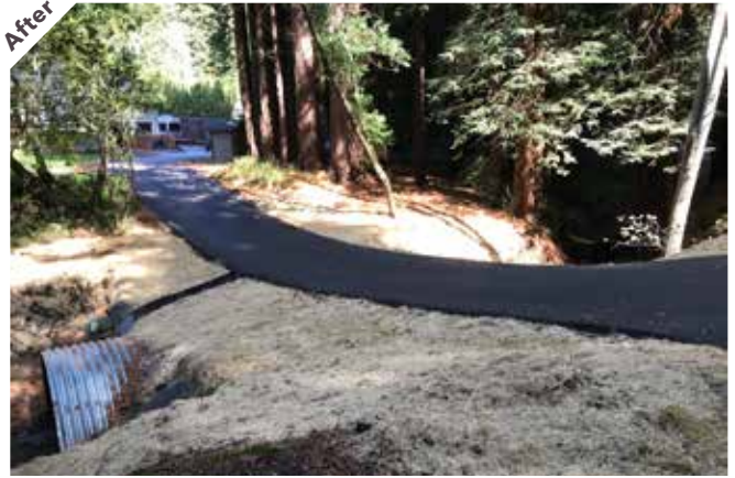
Photo point 1B: Looking upstream at the lower crossing with the new culvert and repaved road.
