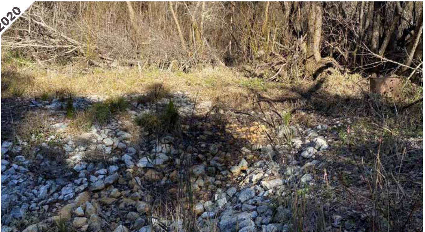
Photo point 1: Looking upstream, the rock-lined open channel that replaced the undersized culvert has become revegetated with willows and herbaceous vegetation.
