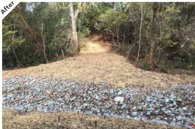
Photo point 3: Standing on the remaining embankment and looking north, the rock lined channel and willow stakes are visible.
