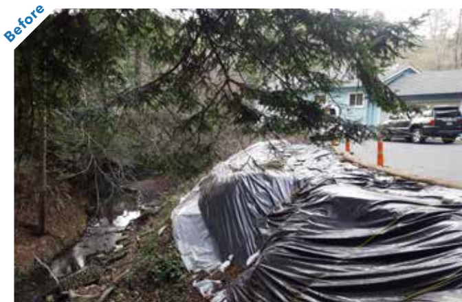
Photo point 2: The eroded streambank covered in plastic can be seen on the right. Branciforte Creek is visible on the left.
