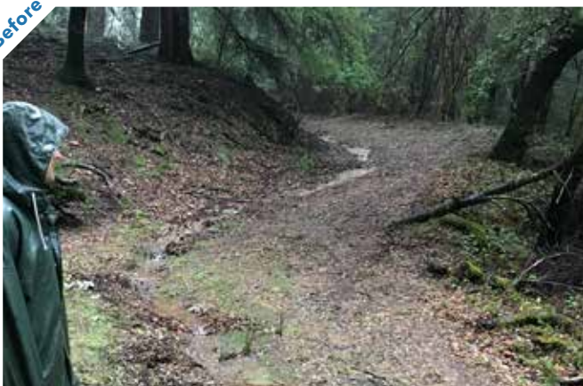
Photo point 9: Looking uphill long the upland portion of the road. The road is insloped the whole stretch above this point with no ditch relief thus contributing to runoff created erosion,
