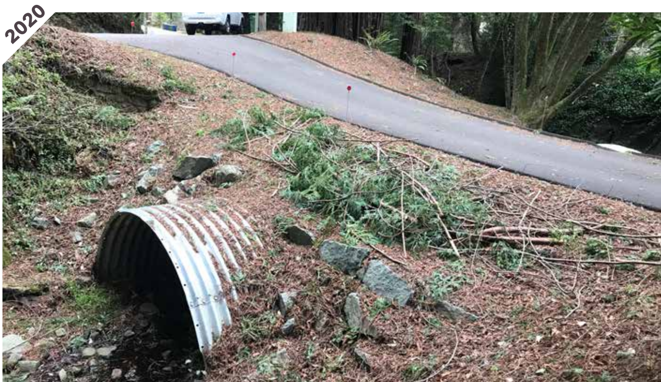
Photo point 3B: There is still no erosion present at the culvert inlet. Banks are stable with a good cover of native duff.
