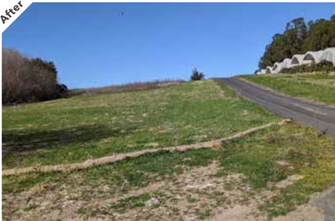
Photo point 4: Looking north, after spoils placement the site has been seeded with common barley and a fiber roll installed.
