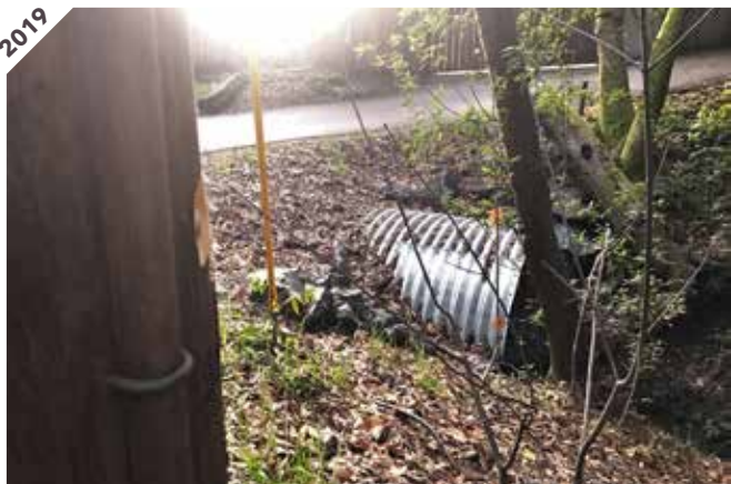
Photo point 3A: The culvert is functioning well and no erosion is present. Note the tree that fell on the right that was partially cut to unblock the road but the trunk was left in place.
