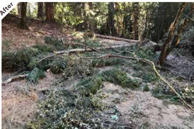
Photo point 9: The road was outsloped to reduce runoff and covered in duff and wood debris from onsite.
