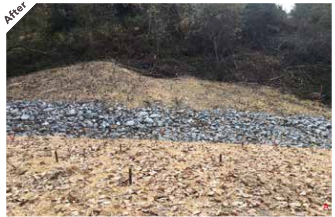
Photo point 5: Standing on the remaining embankment and looking south the culvert has been removed and replaced with a rock-lined open channel.
