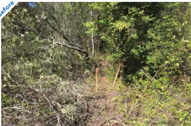
Photo point 3: Standing on and looking north across the failing embankment.
