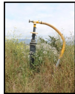
Methane collection pipe
