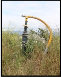
Methane collection pipe
