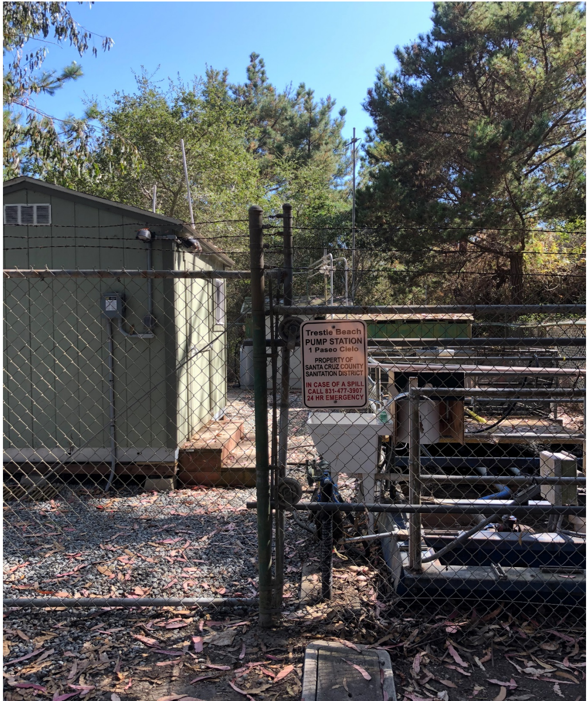
CSA 20 - Trestle Beach Treatment Plant
