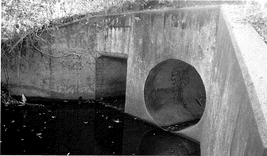
Figure 3 - Existing Caltrans culvert underneath Highway 1, downstream of private twin 48" \varnothing culvert. Photograph taken December 18, 2015, 2:15pm.
