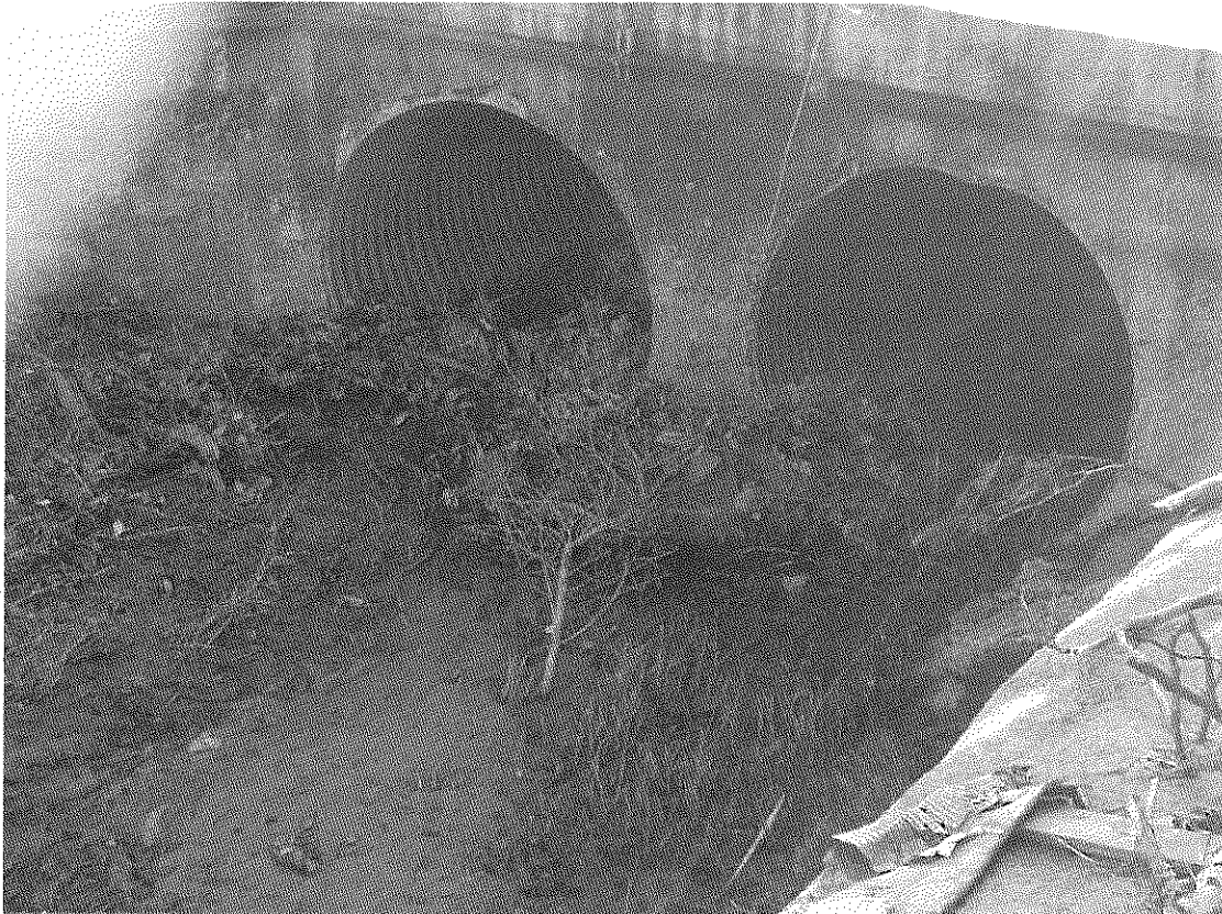
Figure 2 - Existing privately maintained twin 48" Ø culvert inlet located approximately 90 feet downstream of the project property. Photograph taken December 18, 2015, 2:00pm.
