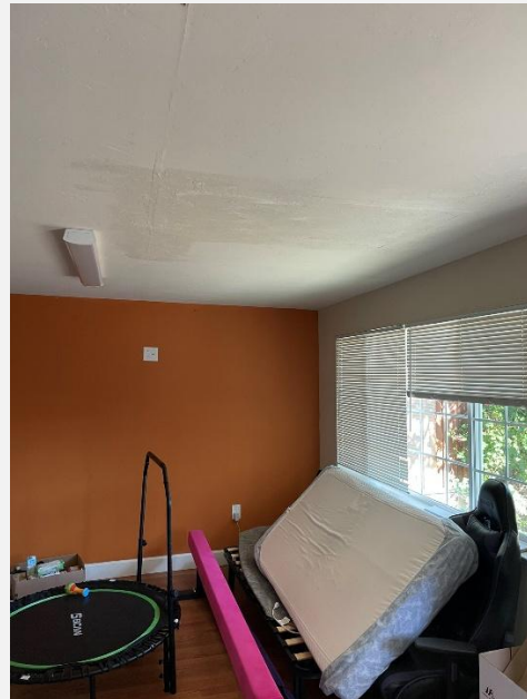
Photograph 26. Photo showing potential water damage on ceiling of single-family residence.
