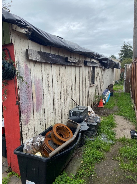
Exhibit 11: Overview of garage structure along south boundary of 2030 17 th Avenue. View E 81°.
